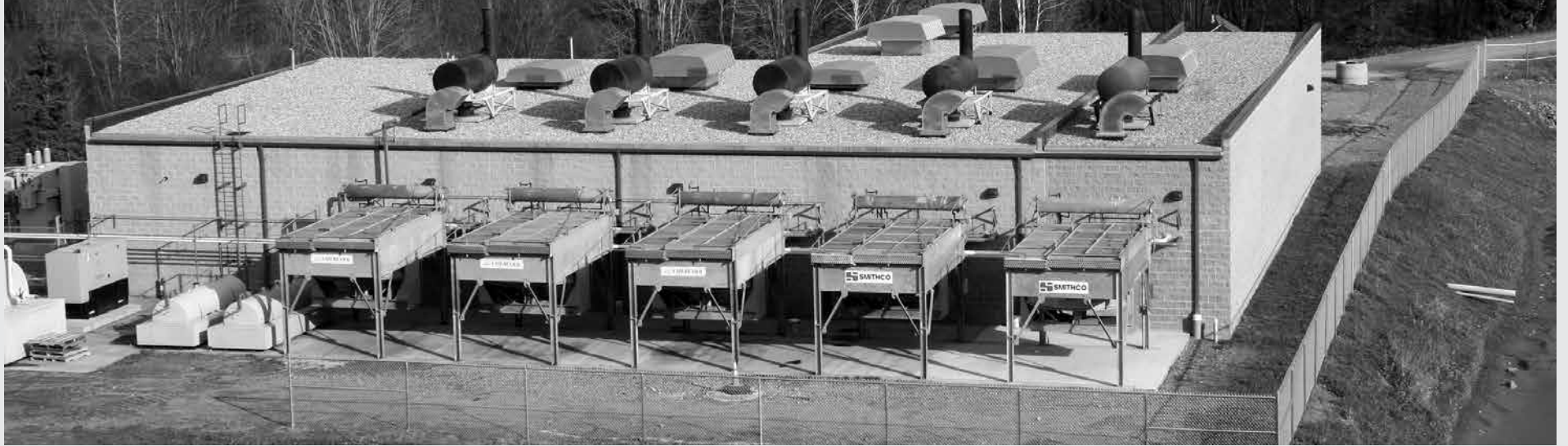
An aerial view of the Coventry Landfill plant from 2009. The plant generates electric power from landfill methane, harnessing a greenhouse gas into a renewable energy resource and supplying WEC members with an environmentally and financially stable electric source.
