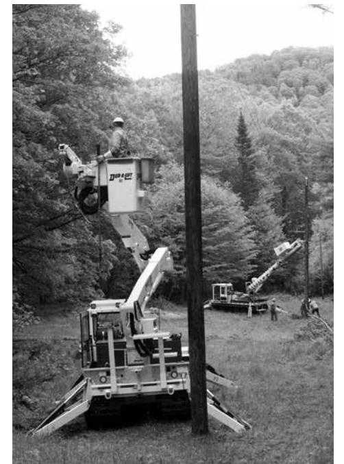
WEC now has two track vehicles, enabling faster and more efficient construction projects in the most rural, off-road territory. Both were at work in the reconstruction project in East Topsham in early June.
