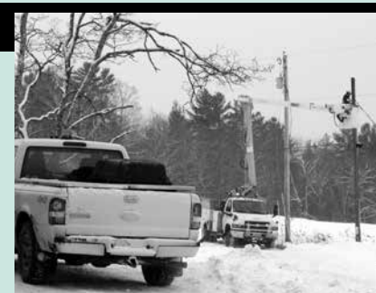
Line maintenance and outage repairs are accomplished more quickly, economically, and safely when the poles and wires are accessible from the road, as in this location (above) in Marshfield. Stories in this issue address the promise, and the problems, associated with that goal. Pages 1 and 4.
